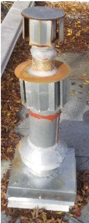
Figure 3: Visual Inspection of Vent Pipe is NOT Sufficient .
