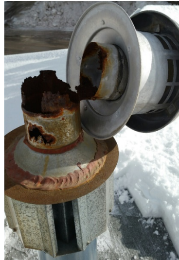
Figure 2: Failed Concentric Vent System
